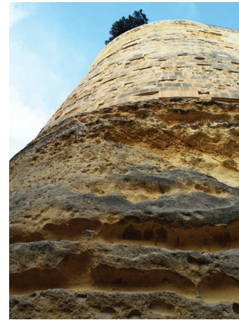
FIGURE 16 The blurred distinction between the naturally formed limestone of the deep outer defensive cut of the Fosso and the ashlar form of the metropolis above.
