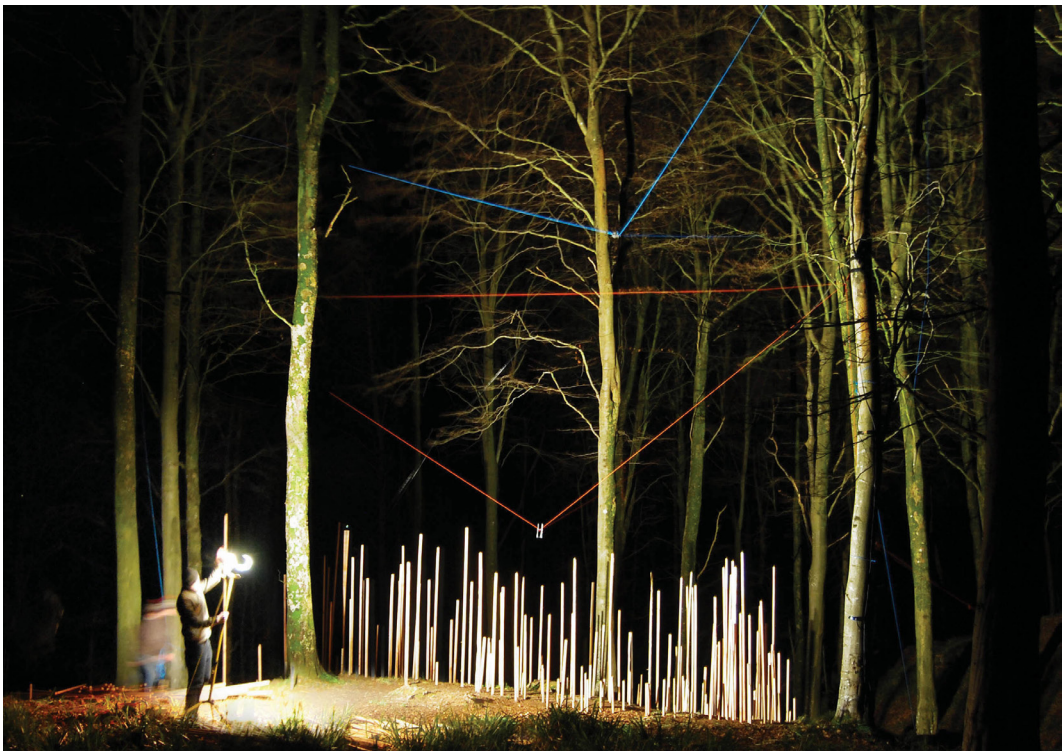
FIGURE 9 Construction and final installation of the field of elements on site, using a web-cam suspended from the trees and a cable robot pointer device.
