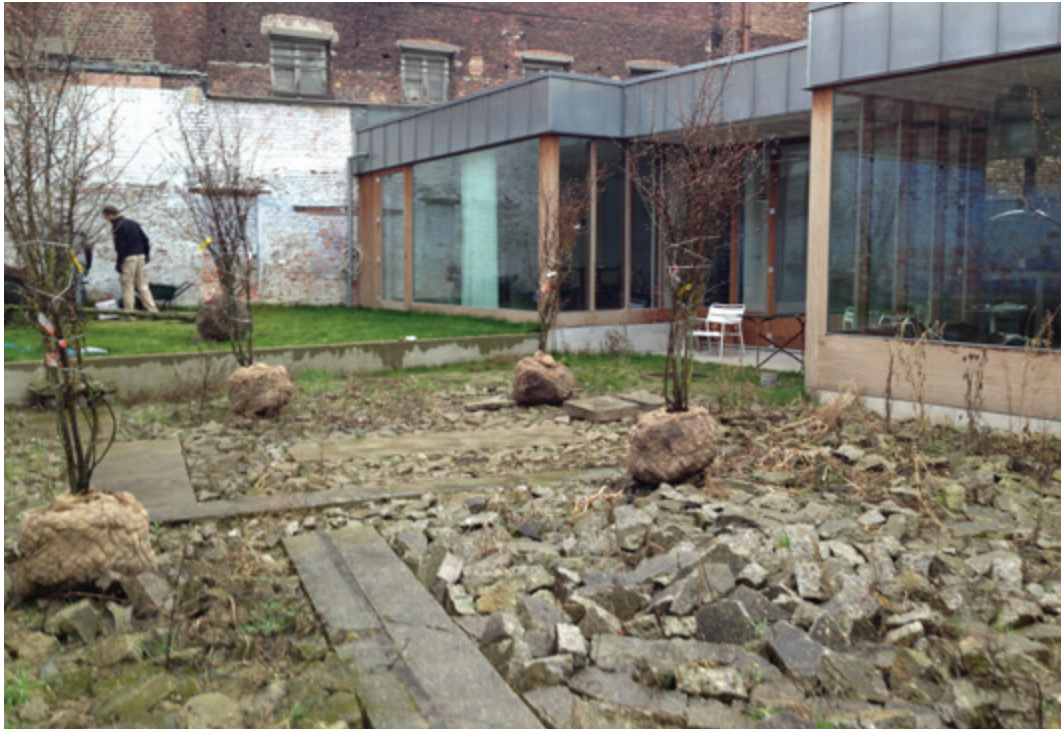
FIGURE 3 Construction of a framework for the different garden zones through differentiated soil treatments. The design of the central garden (bottom half of the picture) literally breaks through the sealed character of the site by scattering the concrete slab into the plant substrate. Several strips of concrete are left unscattered to be used as pathways. The plantings of Amelanchier ovalis ensured the client of the direct presence of structuring green. In the upper garden (top half of the picture), reachable by a concrete step, the concrete slab was fully removed and grass with two Celtis occidentalis was provided. This approach enabled different modalities of floral and human recolonisation and in doing so stimulated a variety of garden experiences. (Photograph by Geert Meysmans, 2013. Reprinted with permission).
