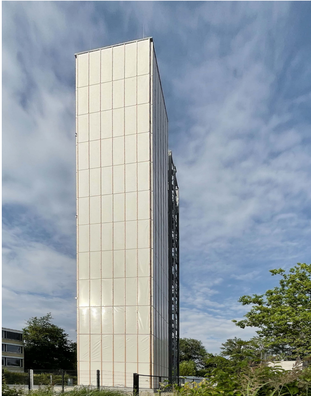
FIGURE 6 Adaptive high-rise under construction on the campus of the University of Stuttgart (© ILEK, Institute for Lightweight Construction and Conceptual Design)
