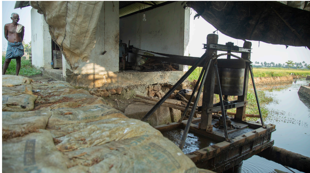
FIGURE 3 The pettium parayum is an indigenous dewatering technology, which runs on electric power, to periodically remove excess water from the paddy fields. (George, 2021)
