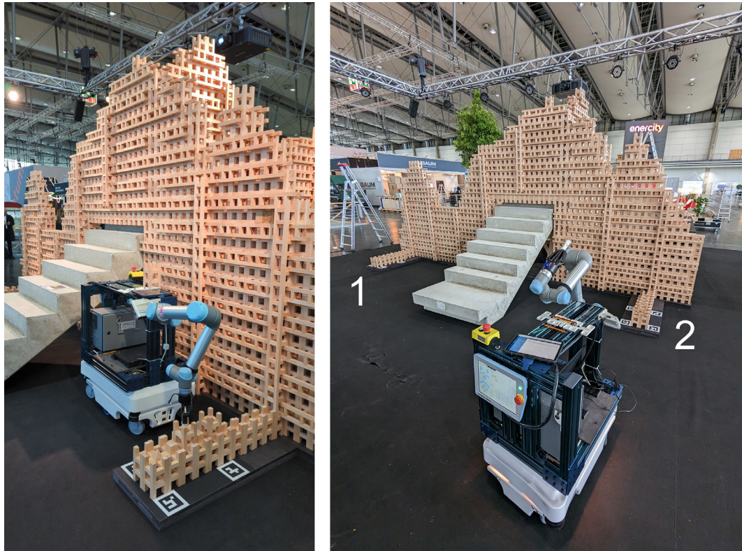
FIGURE 13 MiRo assembling the H-Blocks on-site. In the right image, both material stations are identified. Authors, 2023.
