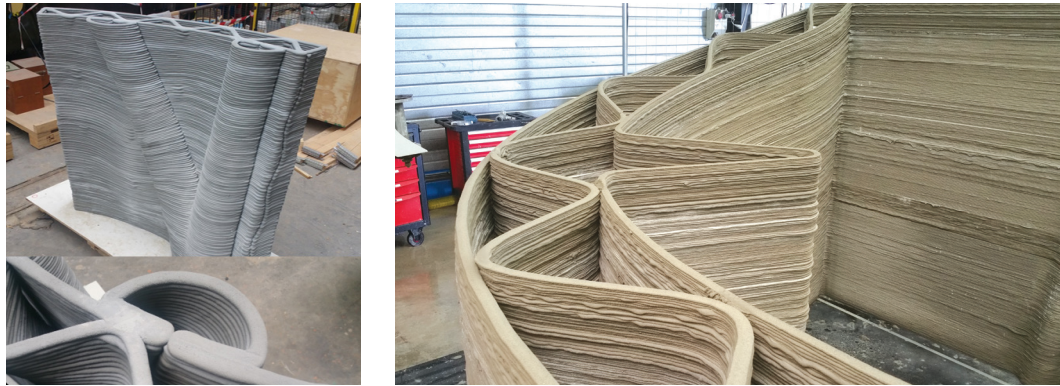
FIGURE 2 UHPC 3D printing. From: C. Gosselin, R. Duballet, P. Roux, N. Gaudillière, J. Dirrenberger and P. Morel, Large-scale 3D printing of ultra-high performance concrete—a new processing route for architects and builders, Materials and Design , vol. 100, pp. 102-109, 2016. and XtreeE, http://www.xtreee.com
